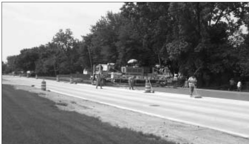
The Six-S crew finishes the four-inch overlay slab on Merriman Road in June, 2003.
