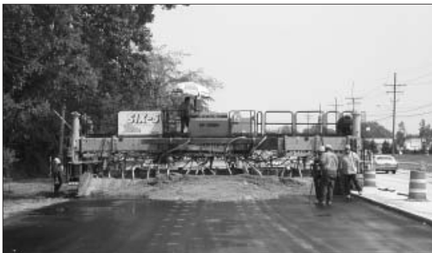
Placement of concrete, including Blast Furnace Slag, supplied by Edw. C. Levy Co., on Merriman Road in Westland, Michigan.
