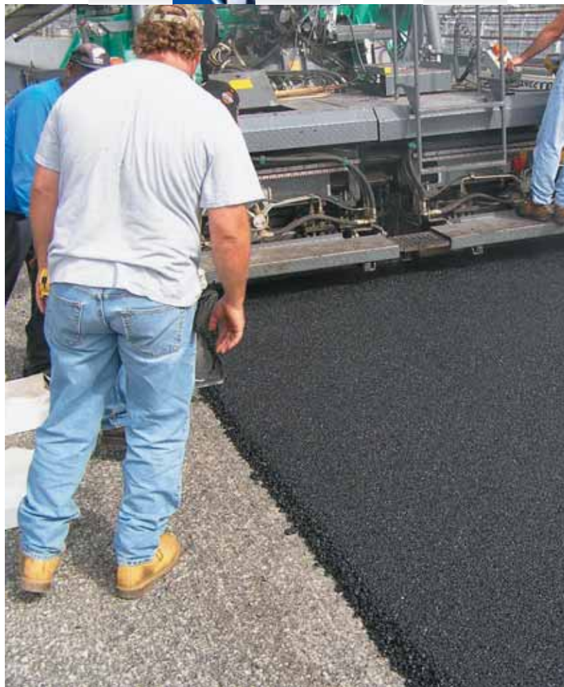
Work crews laid the asphalt mat as close to the retaining wall as possible.
